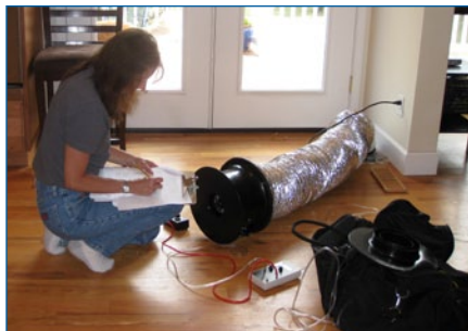
Energy Expert Cathy Cartmill tests a home's duct system. Leaky ductwork can cause air quality problems, uncomfortable drafts and higher heating & cooling bills.
