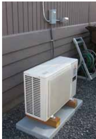
The outdoor unit is connected to the indoor unit by a small opening in an exterior wall.
