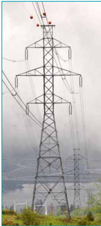
Transmission lines like this one near Rainier carry electricity to substations that serve thousands of customers.
