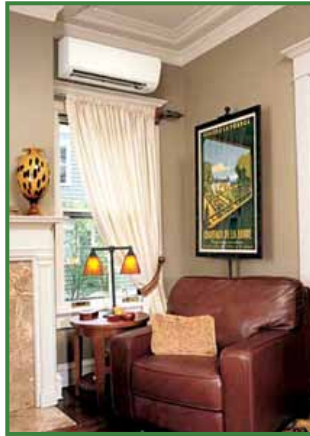
The indoor head of a ductless system sits above a window.
