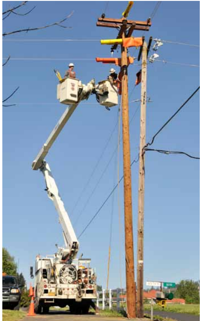
System maintenance and improvement projects, like this one on Fullerton Road in Warren, are funded through operating revenues, not long-term debt.
