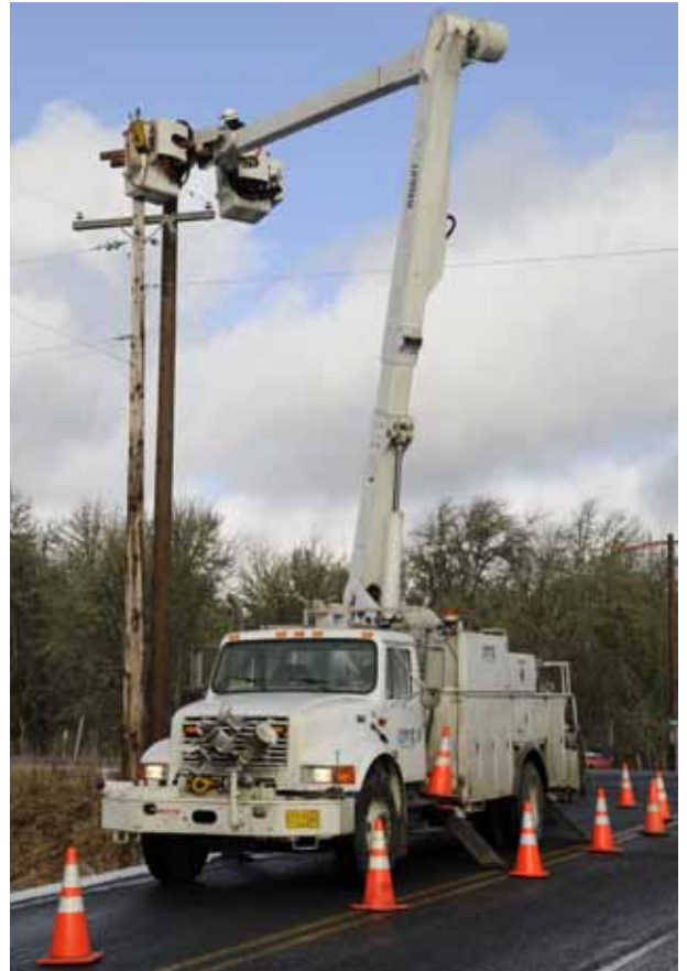
System improvements, like this 2008 project to upgrade a section of line on Heath Road near Rainier, help ensure that we can provide safe, reliable service.
