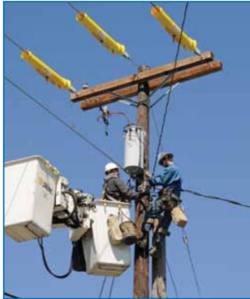
Lineman Cary Gray and Apprentice Jake Feakin replace a utility pole in St. Helens.
