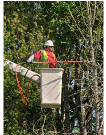
Two crews from Asplundh Tree Expert Company work year-round in our service area, trimming or removing trees and shrubs that are growing too close to the power lines.
