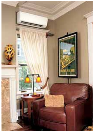
The indoor head of a ductless system sits unobtrusively above the window.
