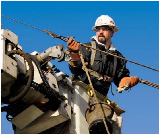
Lineman Cary Gray repairs a power line that was broken when a tree fell through it.
