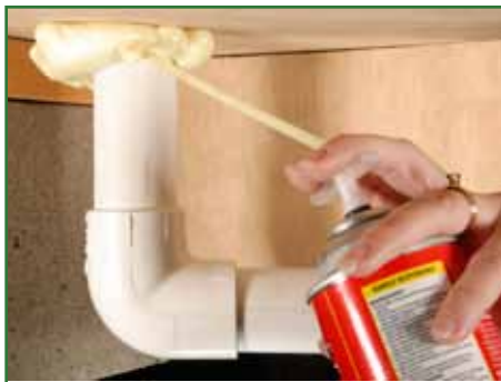
Sealing around plumbing penetrations and caulking & weather-stripping around doors and windows will help keep heat in.
