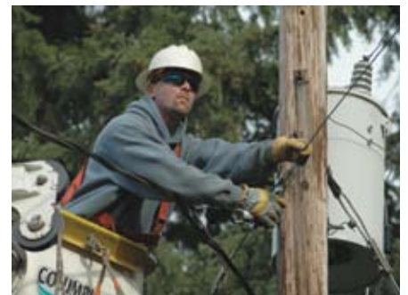
PUD Linemen worked an average of 58 hours each during the first 72 hours after the windstorm.
