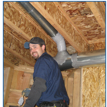
Properly sealed ducts will make your home more comfortable, and increase the efficiency of your forced air heating and cooling system.
