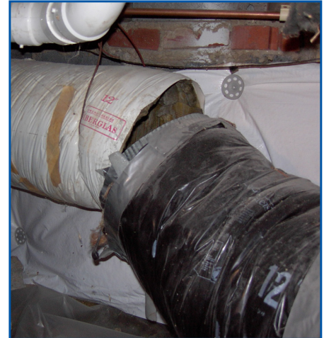
Leaky or disconnected ducts can cause uncomfortable drafts and indoor air quality problems while increasing heating and cooling costs.
