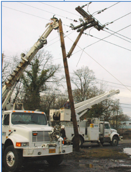
On February 5th a truck hit this utility pole on Pittsburg Road, causing an outage for nearby homes & businesses.
